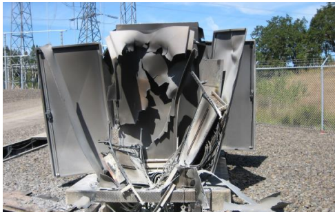
Collateral Damage from Attempted Metals Theft
