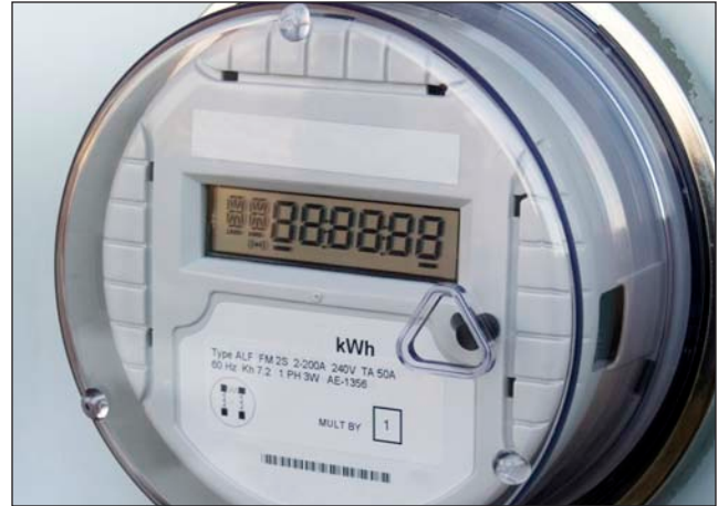
Digital electric smart meter.
