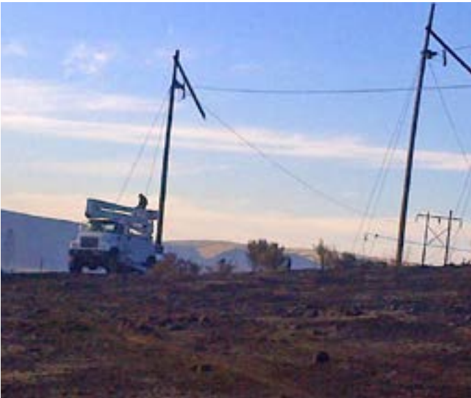
BPA equipment is staged to begin repairing fire-damaged wood poles on the Columbia-Valhalla 115-kV lines near Wenatchee, Wash.
